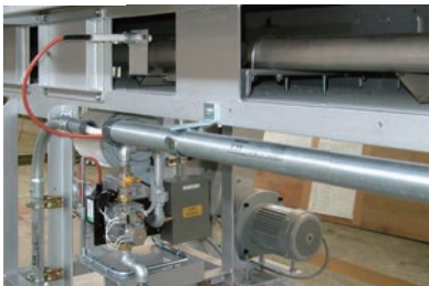
LPG furnace part with metal NIT burner
