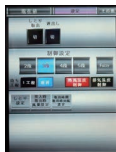
Control setting switching display
